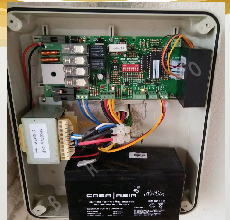
Support backup battery with charging during power failure
